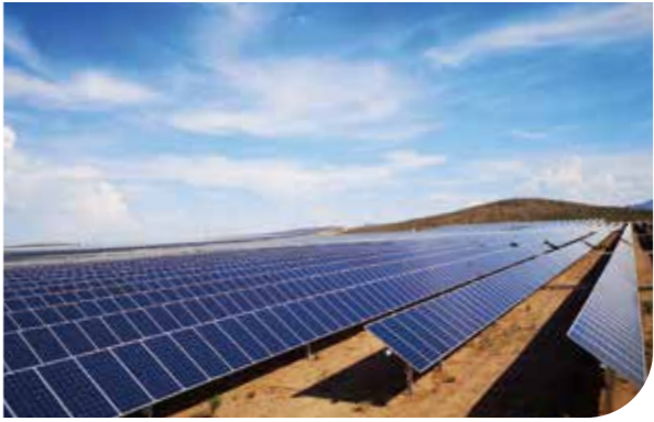
Location: Mexico Capacity: 144MW Technology: SkyLine Tracking System
