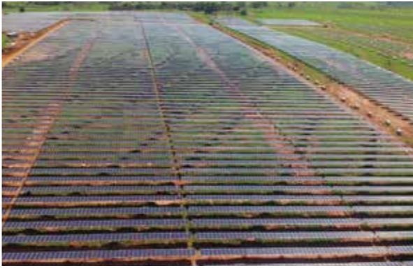
Location: Brazil Capacity: 90MW Technology: SkyLine Tracking System
