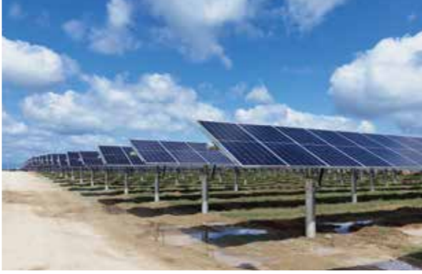
Location: China Capacity: 500MW Technology: SkyLine Tracking System + Bifacial Modules (under construction)
